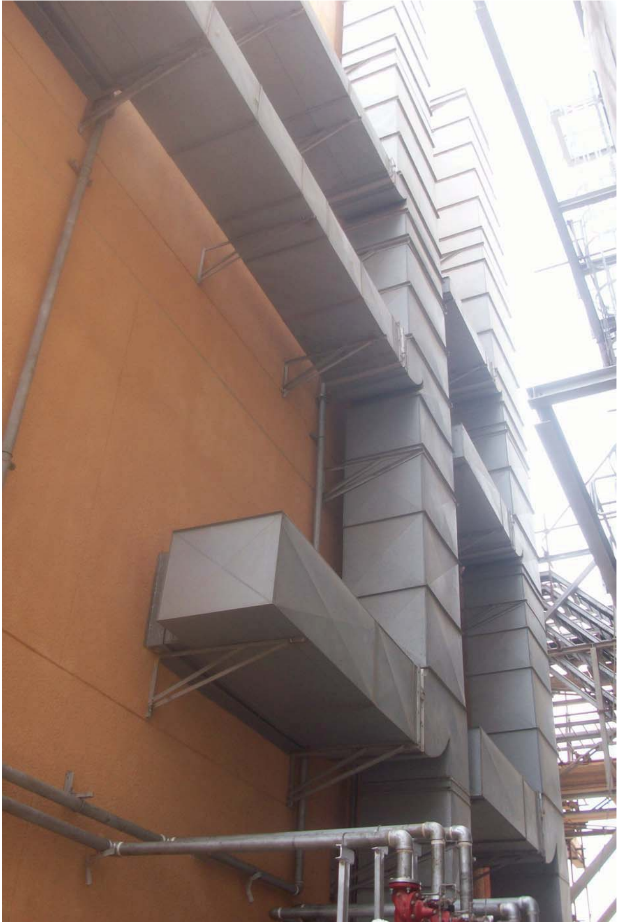
Al Kuraymat Power Plant
