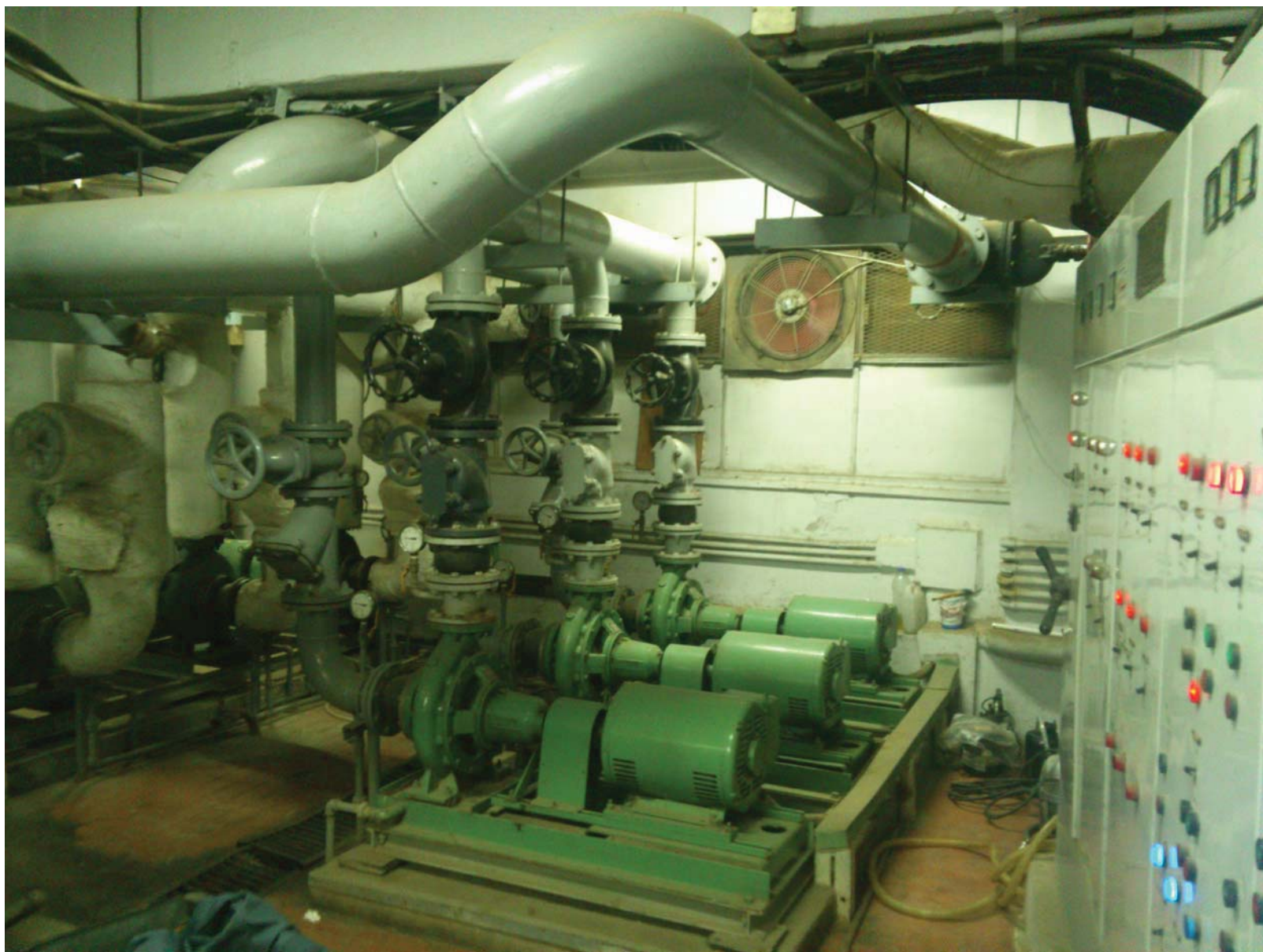
Co-op Petroleum Tower Pumps
