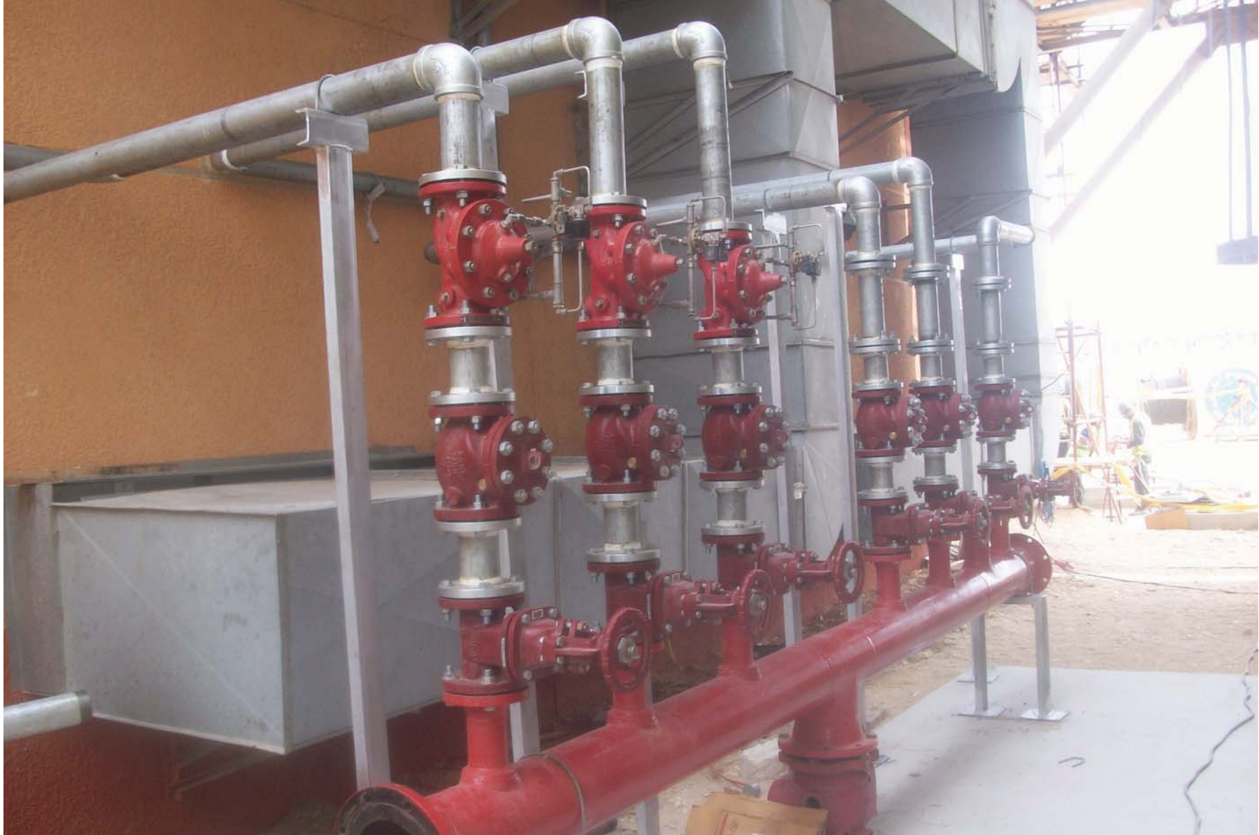
Al Kuraymat Power Plant
