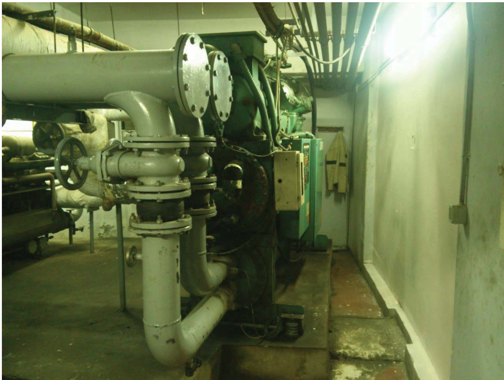
Co-op Petroleum Tower Chiller-1
