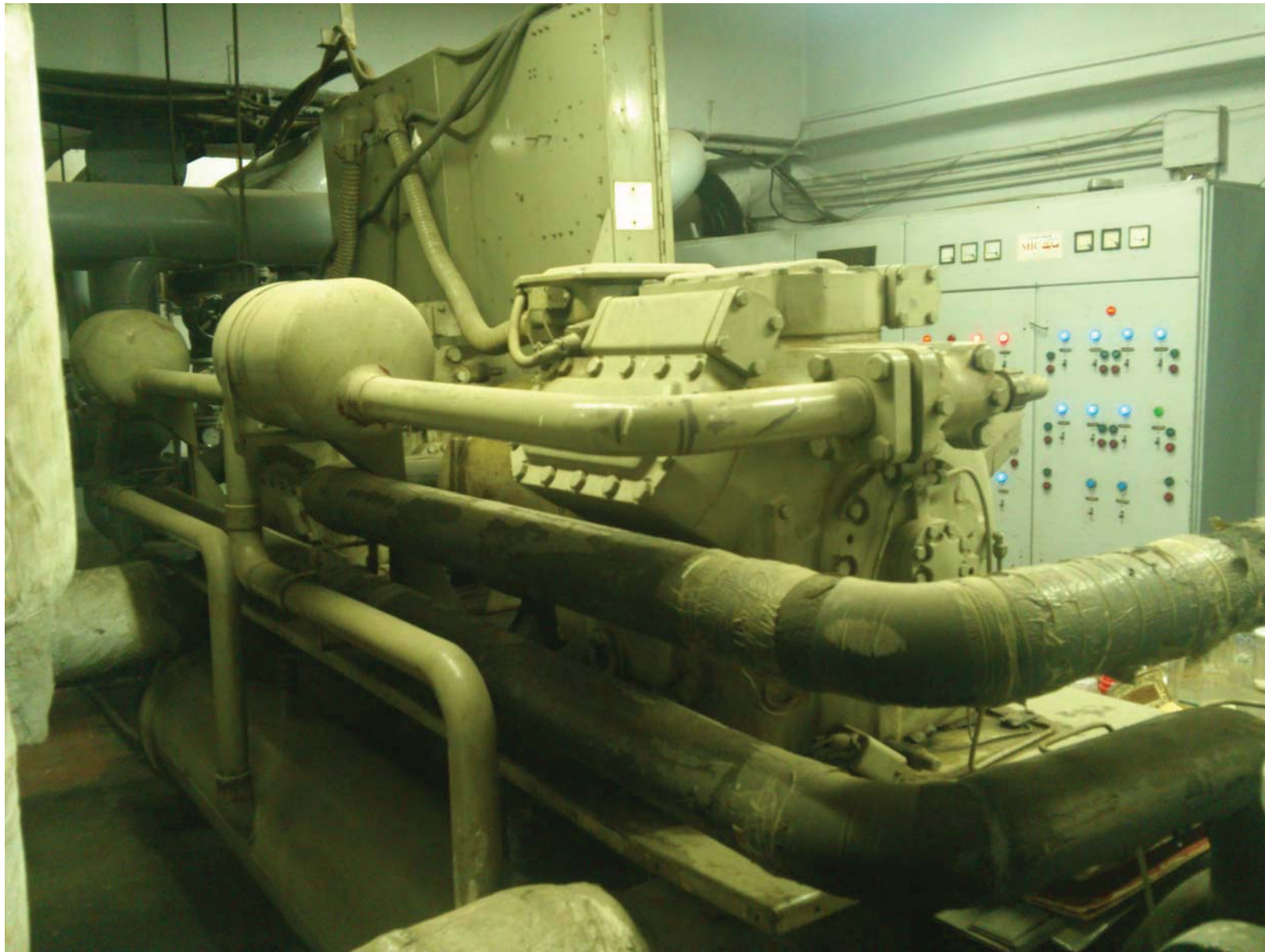
Co-op Petroleum Tower Chiller-2
